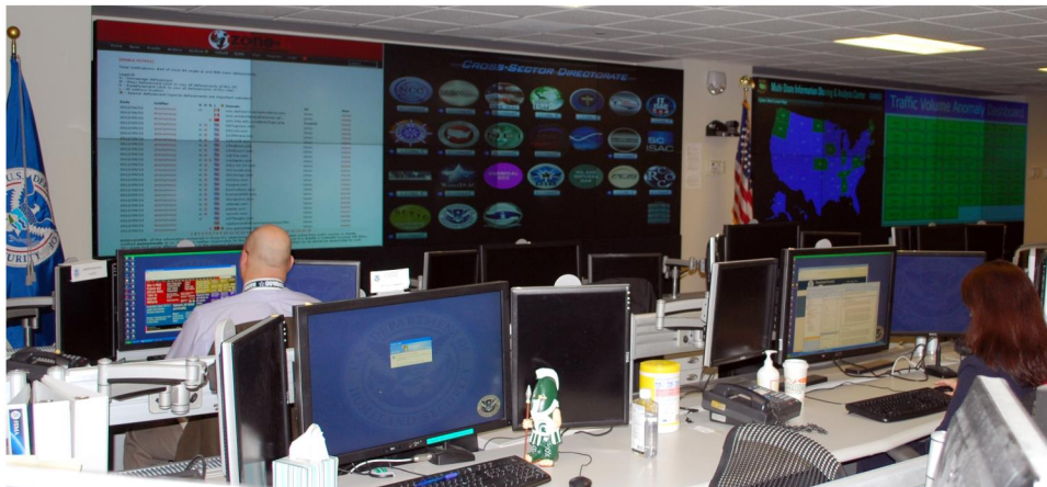
Figure 8: The National Cybersecurity and Communications Integration Center Watch Floor
